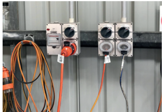
10A to 80A switchgear specified for the manufacturing production area
