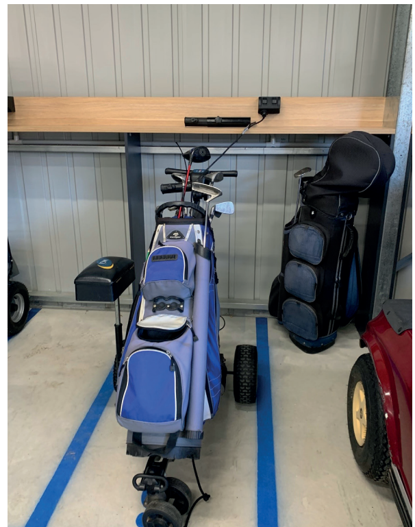
Each bay is powered to recharge battery powered buggies and carts.
